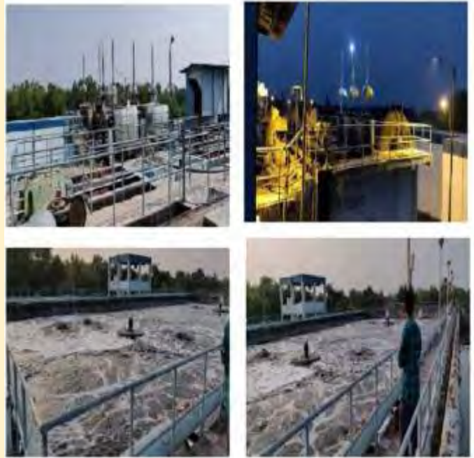
Testing of AHC in STP plant at Nadiad
