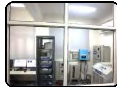
Grid Tied Inverter Test Facility
